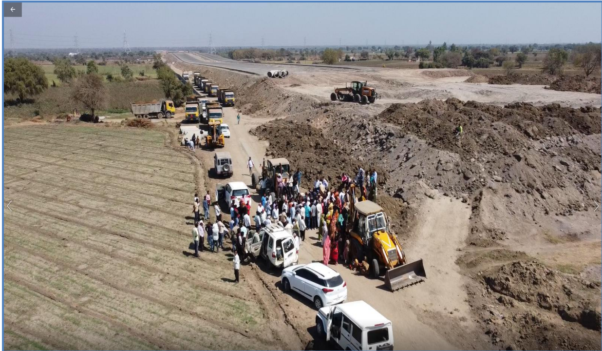
EPC contractor mobilized the manpower and machinery at site with full effort
